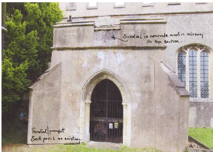
Sundial-parapet as existing (top quarter of sundial missing.)
